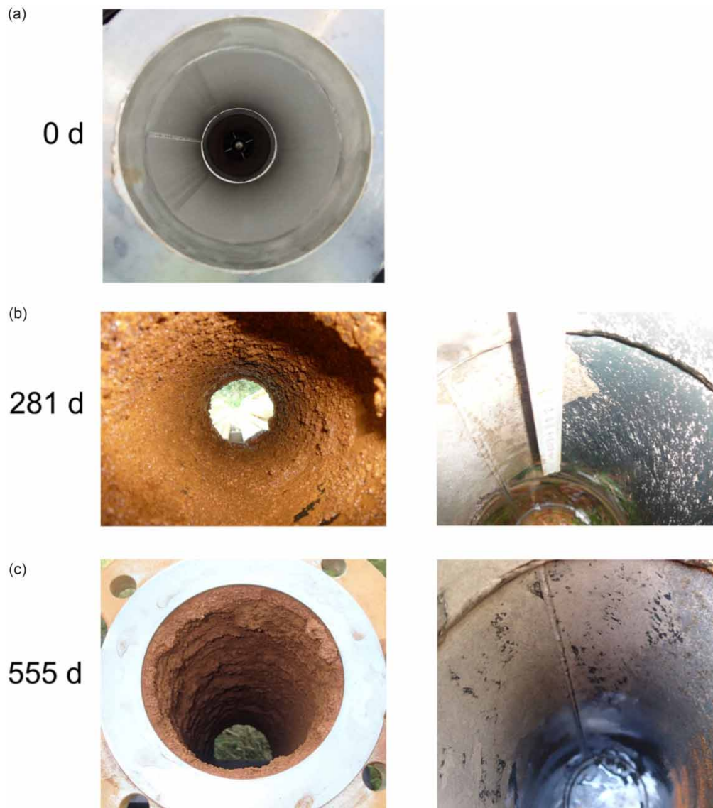
Figure 4 | Riser pipe of Well 7 (silver coating): (a) initial, fresh coating, (b) first inspection after 281 days, left: iron oxide incrustations on inside, right: inside after cleaning, (c) second inspection after 274 further days, left: incrustations on inside, right: inside after cleaning (photographs: Houben, Sander).
