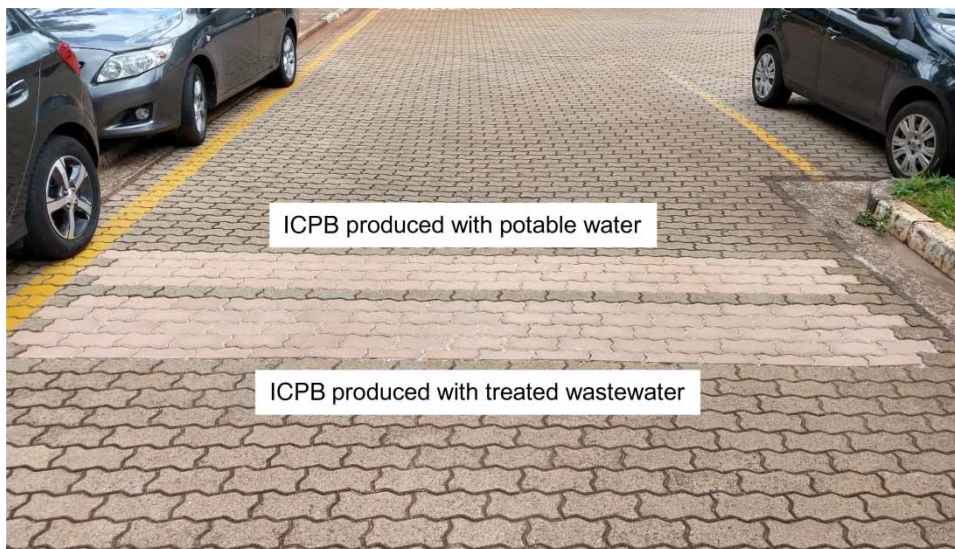
Figure 2 | Interlocking concrete paver blocks (ICPB) produced with treated wastewater and potable water being tested in the parking lot.
