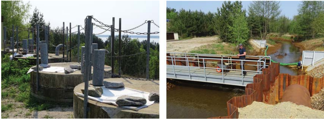
Figure 7.9 Rehabilitation of lignite mines: the case of Lusatia (Germany). Left: groundwater management, right: flooding water channel to fill an open cast mine chain. (Photographs: Petra Schneider )
