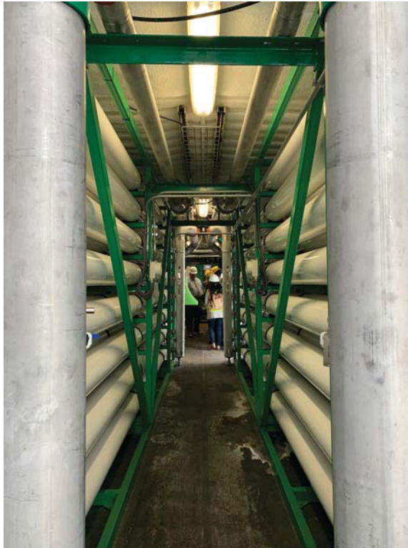
Figure 25.2 Reverse osmosis filtration system is used to treat foundation drainage for reuse at Energy Center San Francisco. Similar smaller systems are used to treat brewery process water for reuse at breweries. (Credit: San Francisco Public Utilities Commission)
