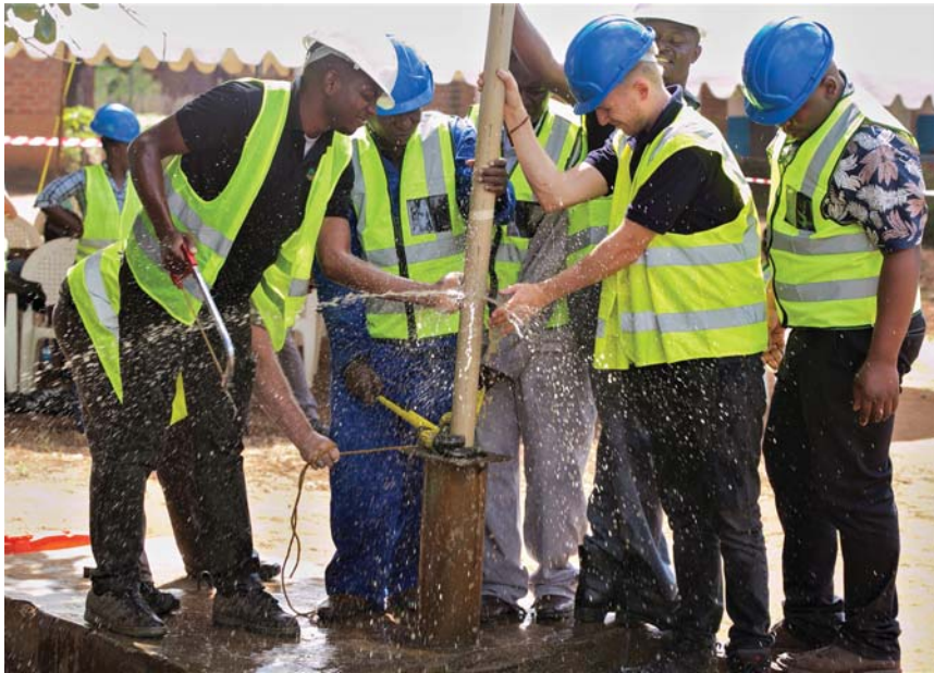
Figure 37.4 Hydro Nation activities in Malawi include capacity building, as in this example of training on borehole installation and maintenance. (Credit: C.JF Water Futures Programme)
