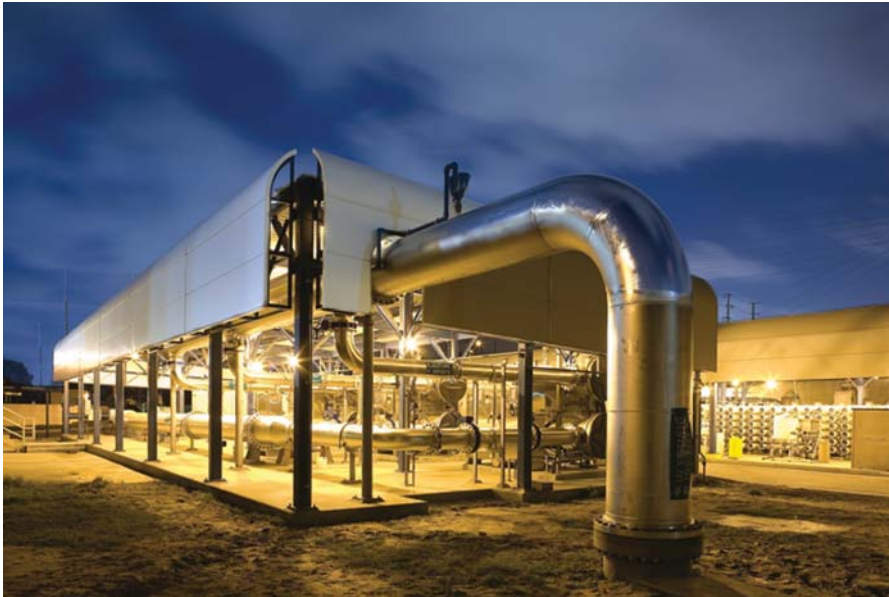
Figure 23.1 West Basin's Edward C. Little Water Recycling Facility (El Segundo, CA) treats 150 ML/d (40 mgd) of secondary effluent to non-potable and potable standards for municipal and industrial reuse. (Credit: West Basin Municipal Water District)
