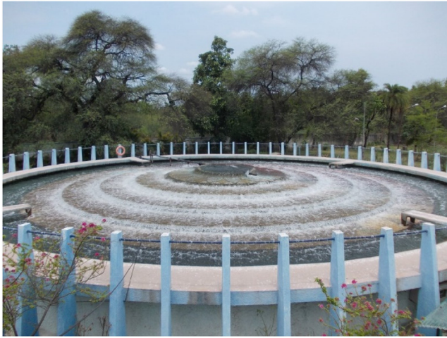
Figure 2.6 Cascade aerator in water treatment plant (courtesy of Nagpur Municipal Corporation and Orange City Water Private Limited, Nagpur, India).
