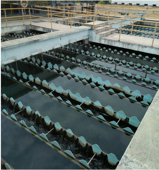
Figure 2.7 Pre-sedimentation tank in a water treatment plant (courtesy of Nagpur Municipal Corporation and Orange City Water Private Limited, Nagpur, India).
