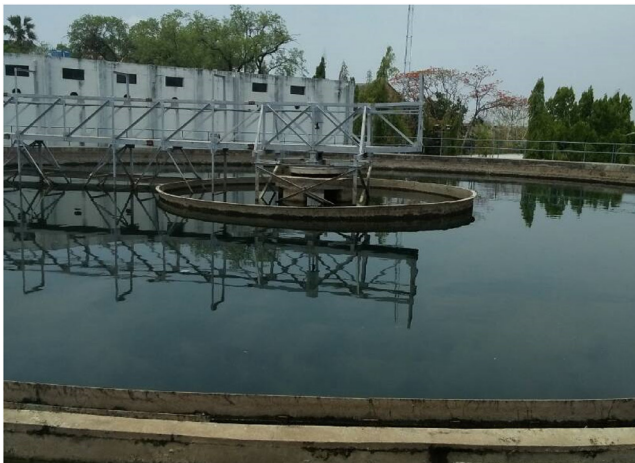
Figure 2.10 Sedimentation tank in water treatment plant (courtesy of Nagpur Municipal Corporation and Orange City Water Private Limited, India).
