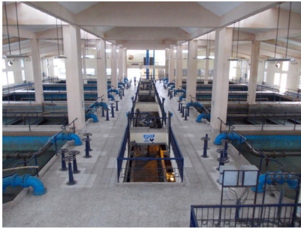
Figure 2.11 Filter house in water treatment plant (courtesy of Nagpur Municipal Corporation and Orange City Water Private Limited).
